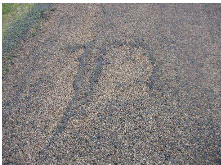
Flush seal over broken pavement Elsiemer Street
